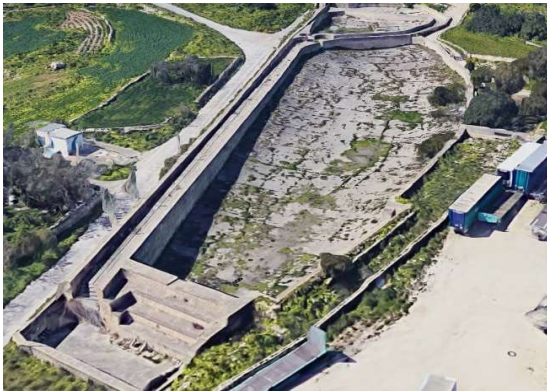
Figure 21: Soakaway at Ħas-Saptan
